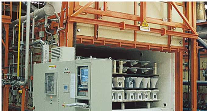
Pressure regulator on excess air burners in the ceramics industry
