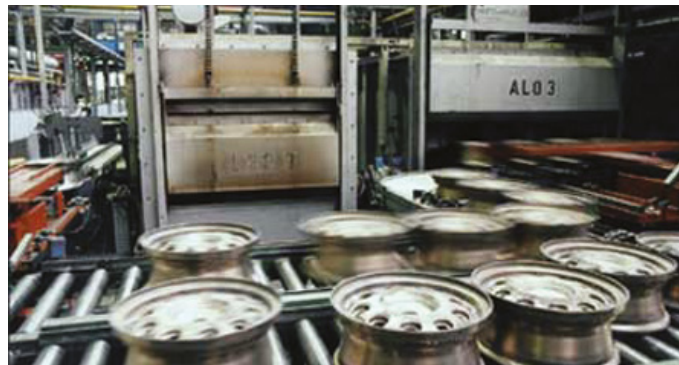
Aluminium age-hardening furnace with air/gas ratio controls for low air pressure protection
